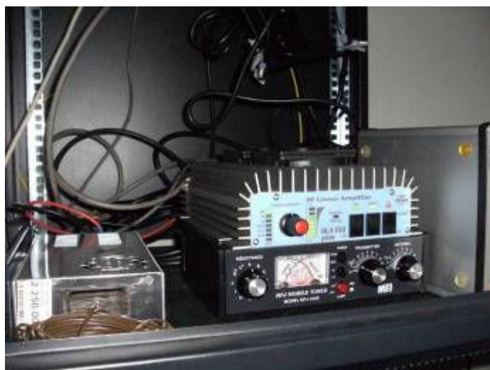
Above: Cabinet with 12V power supply (left) HLA 150plus amp, MFJ-945E antenna tuner (centre) & Zeus ZS-1 transmitter (vertical right)
