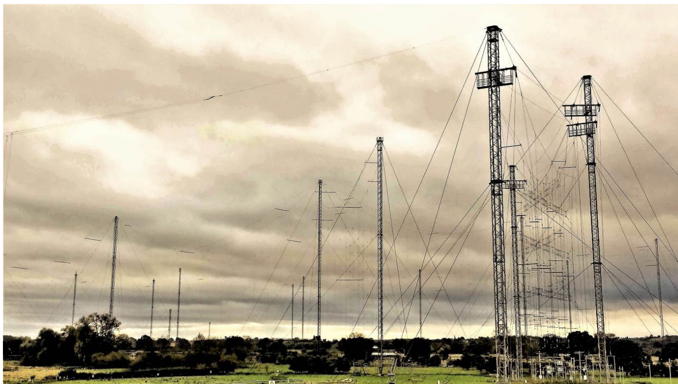
Aerial masts at Woofferton transmitter site, viewed from the east
